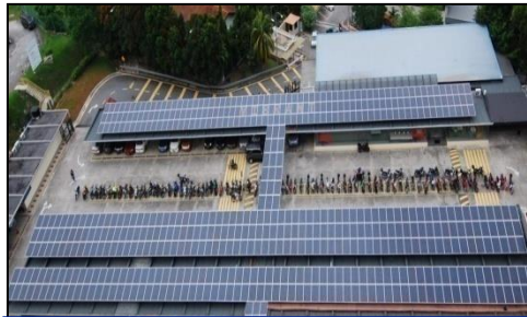
Rooftop Solar PV @ Carpark, TNB HQ, Bangsar
