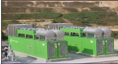
Landfill Gas Power Plant, JV in Puchong, Selangor
