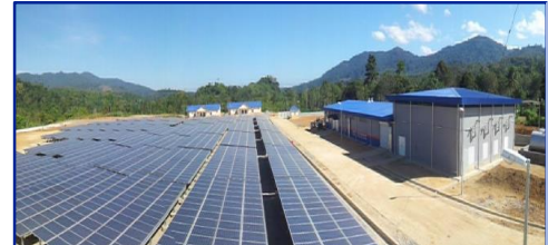
Solar Hybrid System (SHS) RPS Kemar, Perak
